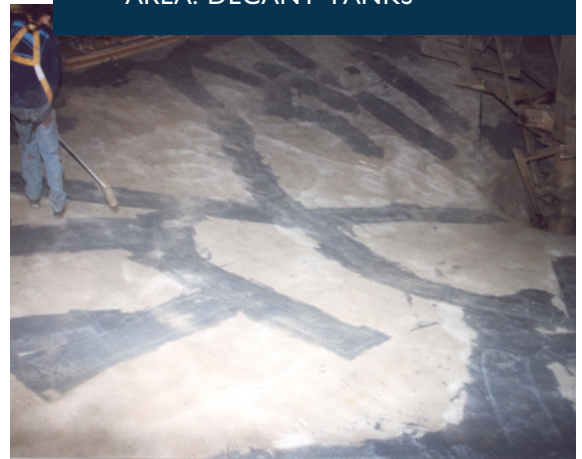
AREA: DECANT TANKS
